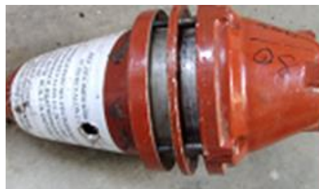
Figure 6. Improper fitting of Spigot joint
