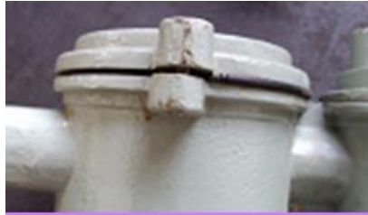
Figure 2. Improper fitting of Gasket in Exd apparatus
