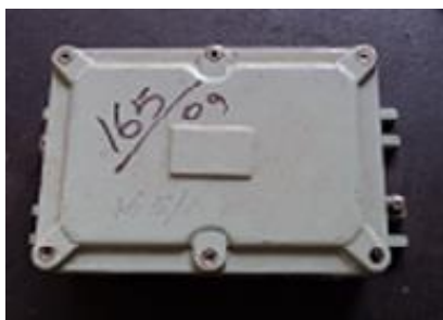
Figure 3. Missing of bolt in the Exd apparatus
