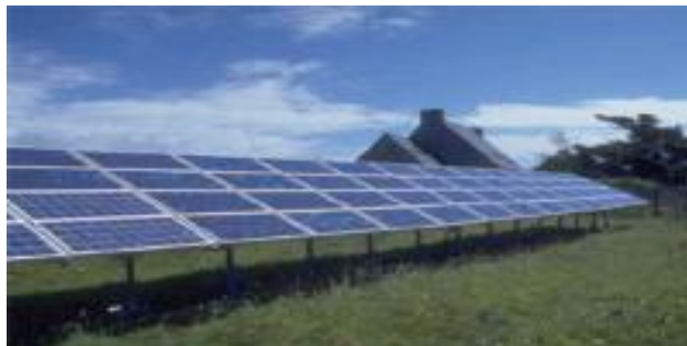
Figure 7. Photovoltaic system solar panels
