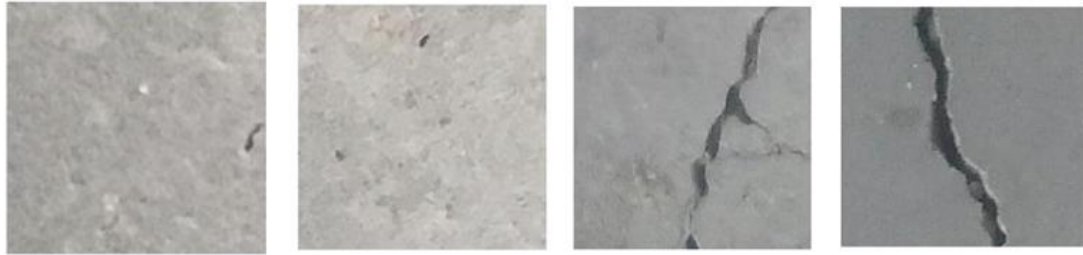
Figure 4. Sample images of concrete surface
