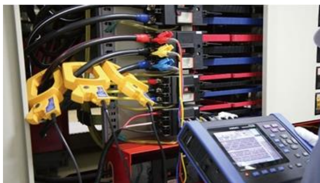
Figure 2. Power Quality Monitoring at CVD
