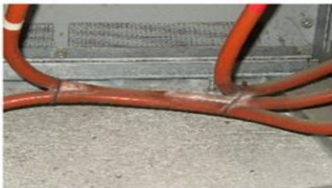
Figure 5. Dust Deposit on Tie-Wrapped Cables [18]
