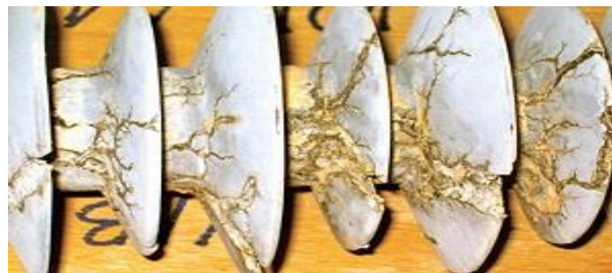
Figure 4. Severe tracking on EPDM sheathed arrester in Oman. Insulator Performance Resolving
