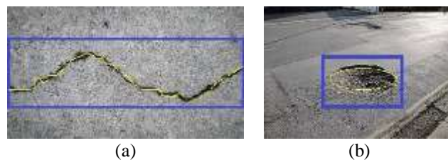
Figure 8. Classification representation of pavement health conditions such as (a) transverse cracks and (b) potholes using the proposed YOLOV8 enabled PavementHealth 4.0 framework
