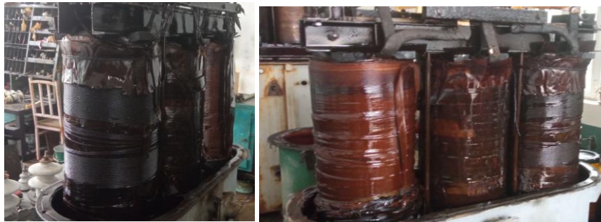
Figure 2. Damaged power transformers detected during the experiment
