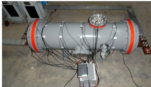
Figure 7. Experimental Set-up of the 126kV Three-phase GIS Bus Bar
