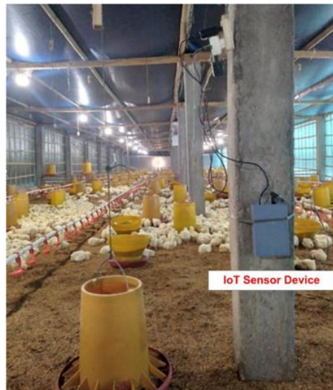
Figure 2. IoT sensor setup installation inside broiler house
