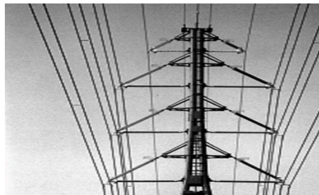
Figure 5. Front view of a compact tower [8]
