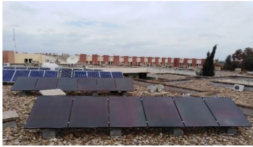
Figure 1. Beni Mellal PV plant
