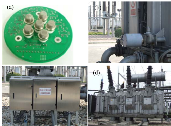
Figure 3. The Photographs of (a) Gas Sensor Array, (b) Transformer Drain Valve, (c) Onsite Control Box and (d) Power Transformer
