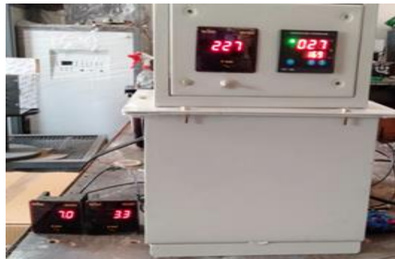
Figure 8. 1.1 kVA, 220/110 V, 10A, 50 Hz, distribution transformer
