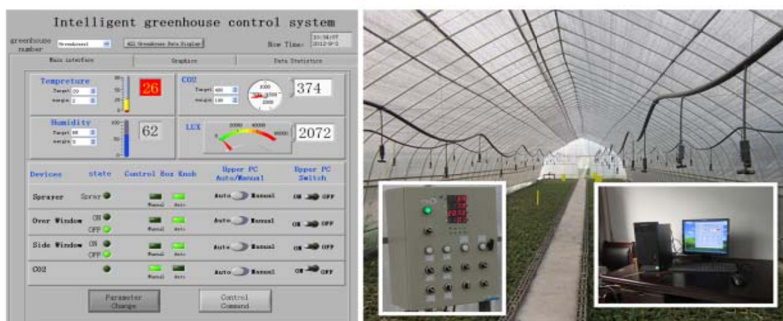
Figure 7. Photo of the Human Machine Interface, Equipment and Working Field
