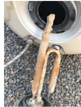
Figure 2. Damage in the water heater causing electrical leakage in the water network
