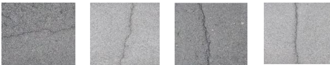
Figure 7. Examples pavement crack images capture using the image acquisition system.
