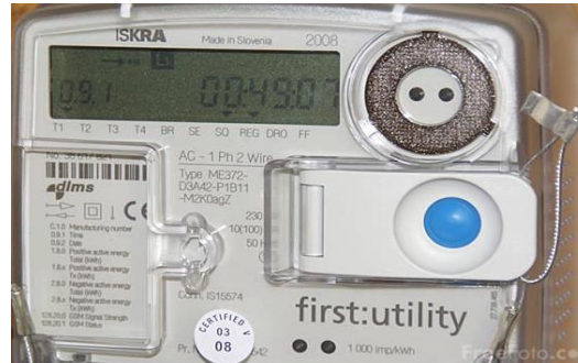
Figure 2. Smart Power Meter
