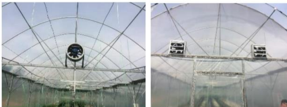
Figure 4. Axial fan (left) and exhaust fan (right) arrangement in the greenhouse
