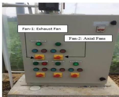
Figure 5. Control Panel located inside the greenhouse
