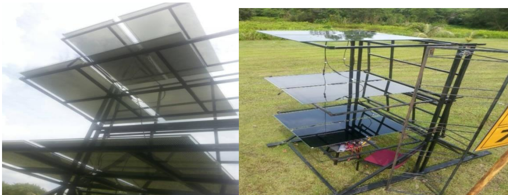
Figure 1. Thin film solar PV panels installed in the UPM University.
