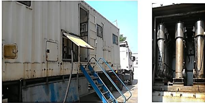
Figure 2. Online Mobile Insulating Oil Reclamation Plant: (left) Mobile Truck; (right) Column Tanks Filled with Adsorbent.
