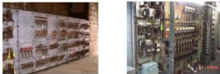
Figure 1. Equipment Designs in 50s and 60s
